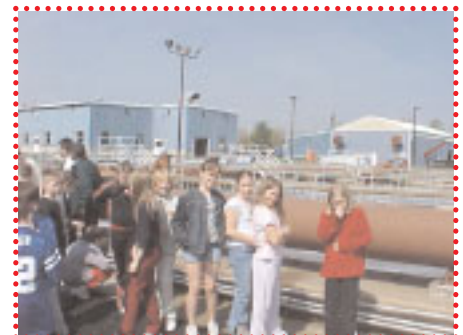
Behind the students at upper-right is piping for the aeration basins where helpful bacteria break down sewage.
