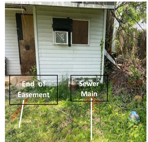
A shed on concrete with electric on the sewer main & easement – a violation of Authority easement restrictions.
