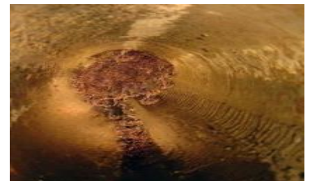
Root intrusion through a joint in the sewer main
