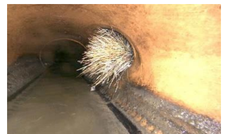
Root intrusion from a service lateral connection
