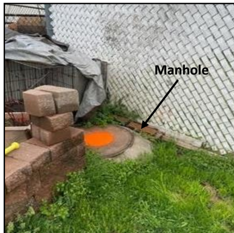
A 24-hour 5' unimpeded access radius around the manhole is required. Pictured above is a direct violation of that requirement
