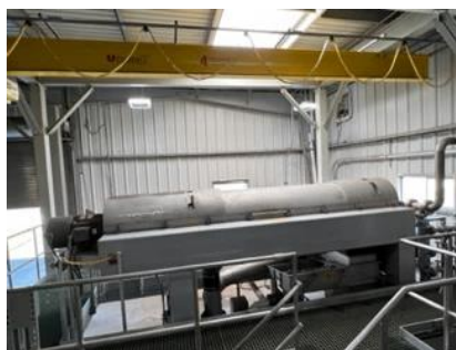
Sludge dewatering centrifuge
