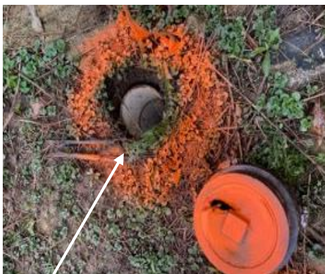
Vents/cleanouts are required to be a minimum of 6" above grade & watertight down to and including service lateral. Above is currently acting as a yard drain and allowing stormwater into the sanitary sewer which is a violation of the Clean Water Act.
